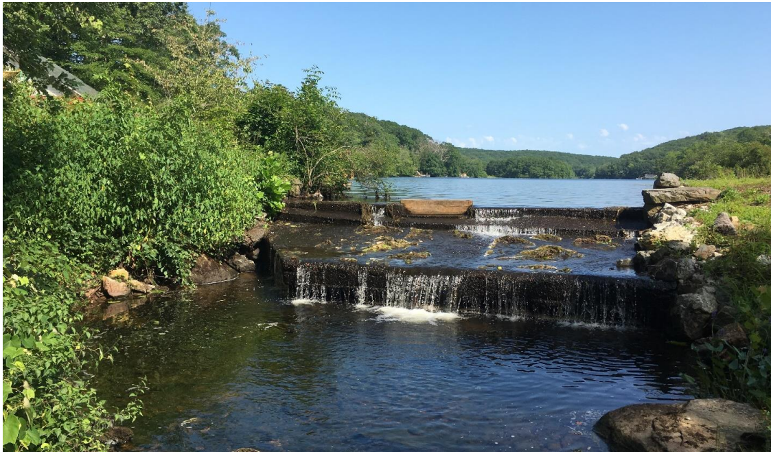
2 - Long Pond Dam inhibits migratory fish access to the natural deep water pond habitat above.
