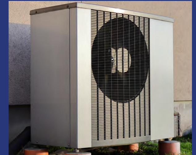
Air-Source Heat Pump (ASHP)
