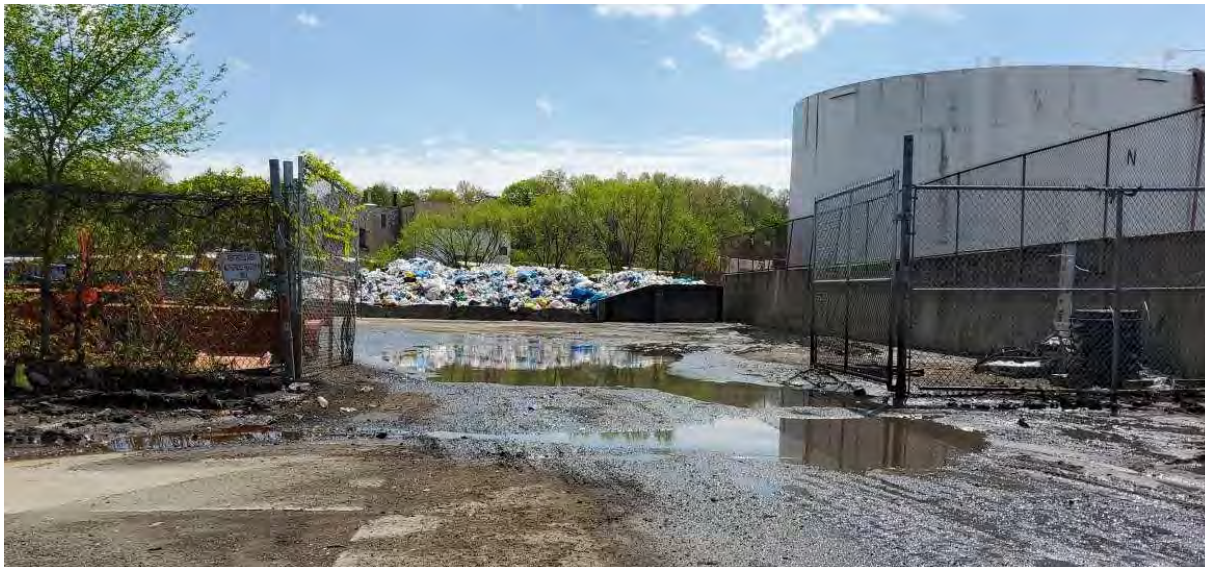
Figure 19. Hotspot Location in the Hutchinson River Watershed: Overflowing Bulk Material Storage and Sediment Accumulation (Mount Vernon)
