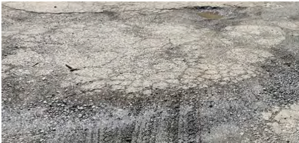
Figure 6. Unmaintained Pavement with Accumulating Debris
