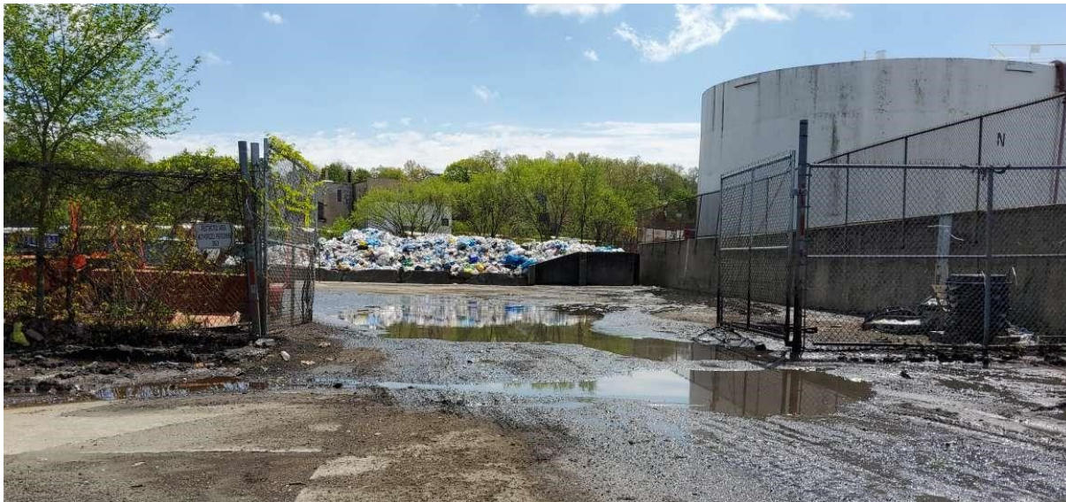
Figure 19. Hotspot Location in the Hutchinson River Watershed: Overflowing Bulk Material Storage and Sediment Accumulation (Mount Vernon)
